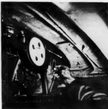
Scrape any traces of carbon from the flange pads and install NEW gaskets using silver paint as a gasket seal.
